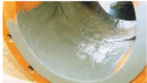
The daily repair routine when epoxy ceramic compounds are used for linings. No hydraulic engineer wants to see irregular surfaces like this ...
